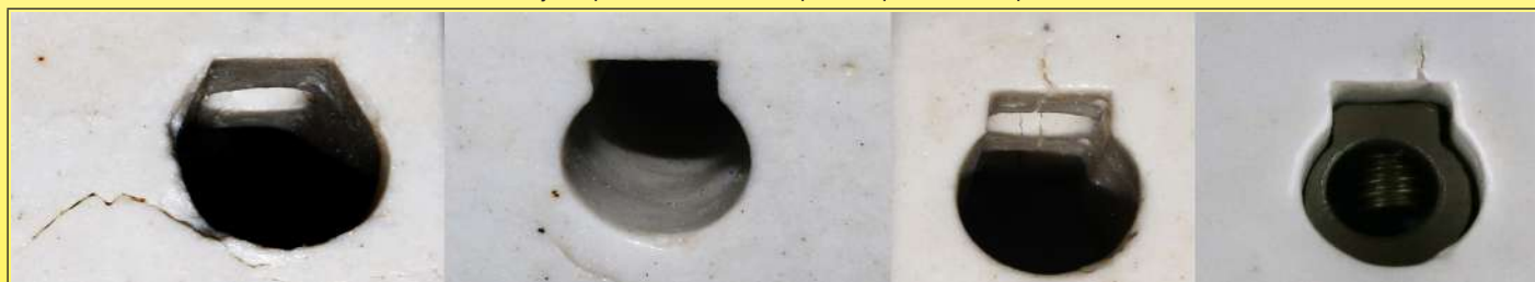
Examples of cracks on C111 porcelain
